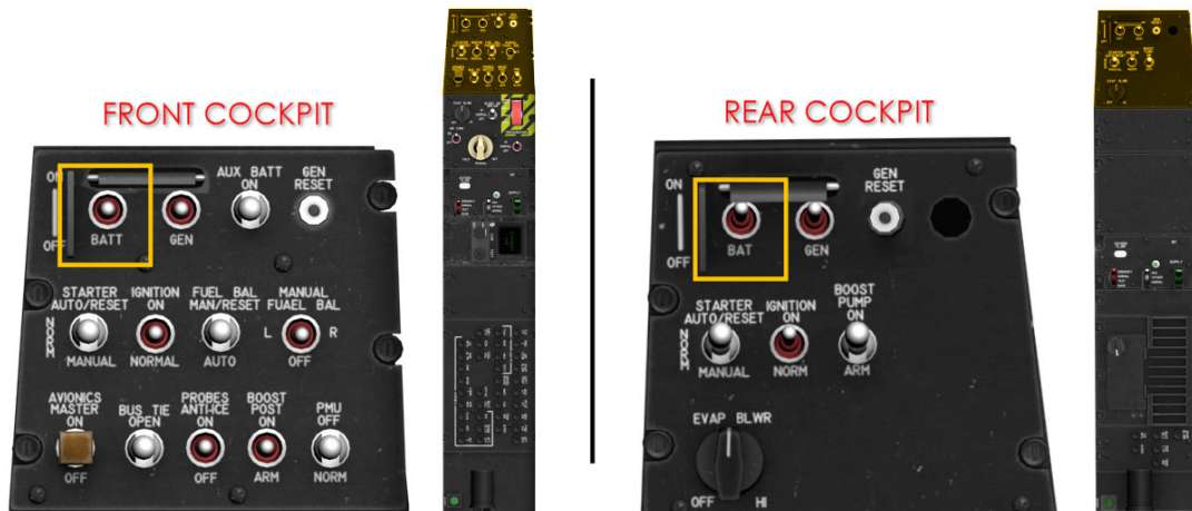
Figure 1-14 Battery Switch Location/s
